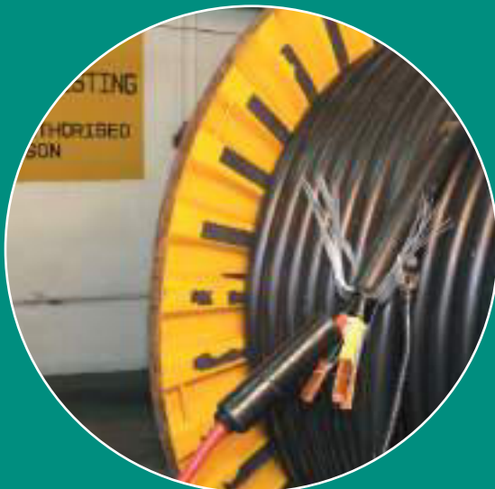
Electrical Test Equipment - High Voltage Test
