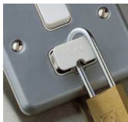
When servicing or repairing appliances fuse carriers on connection units can be padlocked for additional safety
